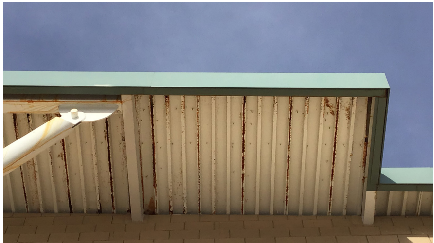
Existing soffit around the leisure pool is showing signs of corrosion and needs to be repaired.
